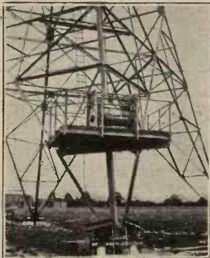
This close-up was taken at Brookmans Park, and shows the foot of one of the London masts, with the winding gear for raising and lowering the aerial.
