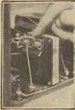
Reversing the primary connections of an L.F. transformer often cures L.F. instability.
