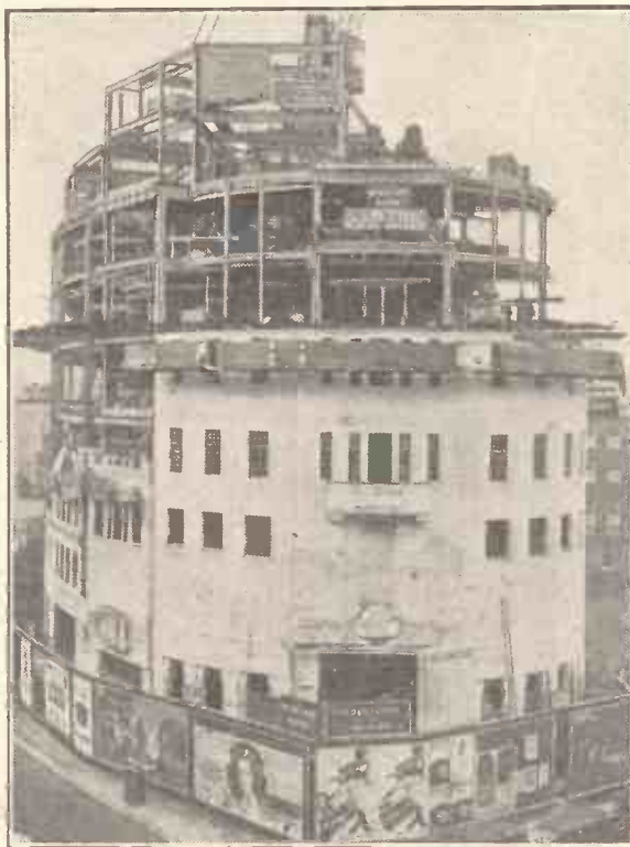
The new B.E.C. Headquarters building is at last beginning to reveal its form and it won't be long before the main constructional work is completed.
