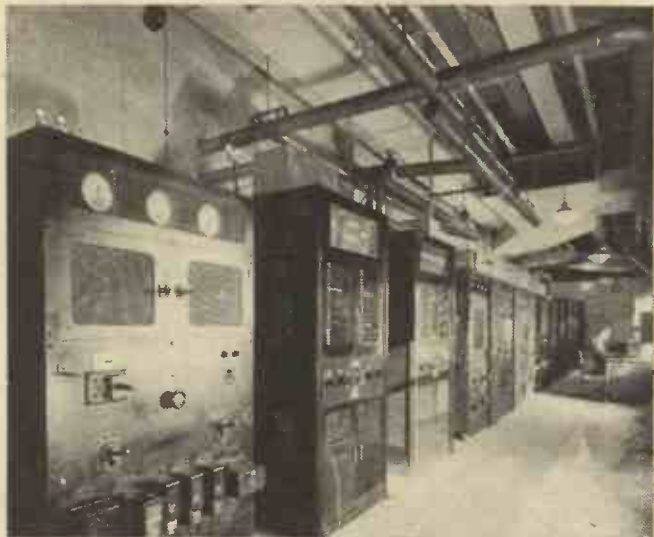
A general view of the R.C.A. television transmitter in the Empire State Building, New York. The pipes near the ceiling are not connected with ventilation but with the feed system to the aerial.
