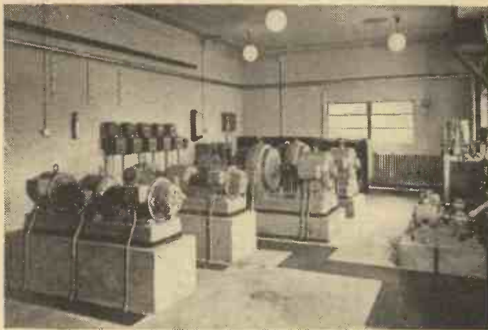
The filament and G.B. generators in the machine-room at Penmon, Anglesey. Both machines are duplicated in case of breakdown. On the right are pumps for water cooling the anodes of the transmitting valves.
