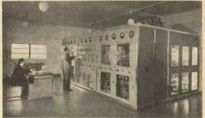
The transmitter and programme control desk at Penmon.
