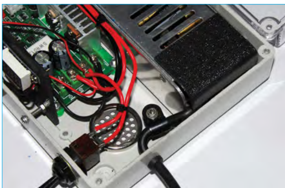
Connections for mains power (top right) should be covered by an insulating shield, as shown here.
