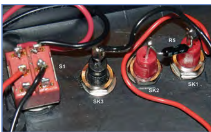
Fig.1.21. Rear panel wiring
