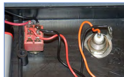
Fig.2.20. Rear panel wiring
