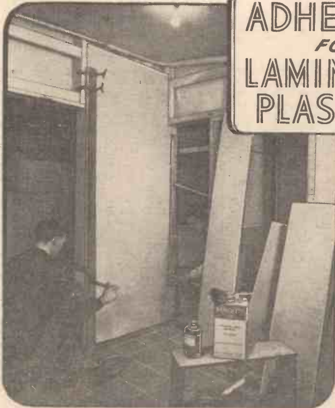
Fig. 1.—A synthetic resin adhesive being used for in situ fabrication. Note the method of using G cramps and wedge struts. (Photo by courtesy of Thomas De La Rue & Co. Ltd.)
