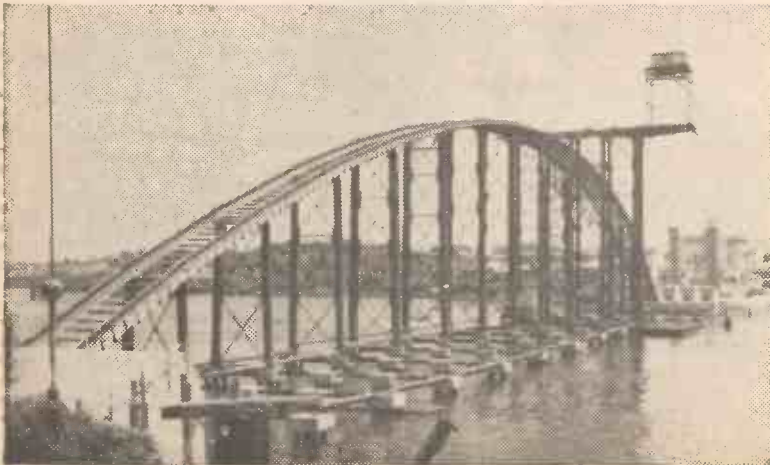
Photograph shows:— Work in progress on the Gladestville bridge across the Parmetta River, Sydney, Australia. When completed this will be the largest pre-stressed concrete span in the world. The steel framework in this picture will support the concrete bridge which is being built at a height that will ensure the free passage of colliers proceeding to and from the Mortlake Gas Works.
