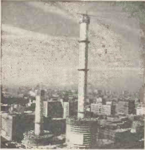
Marina City under construction. The central service cores pass through circular floors; here partly built.
