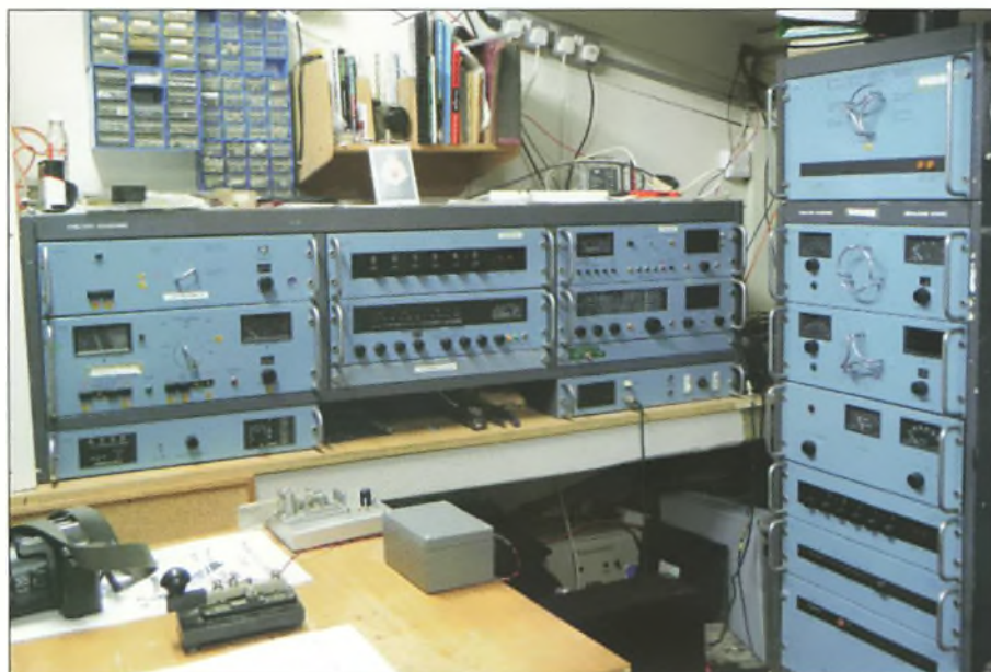
Fig. 3: Kelvin Hughes radio room from RFA Orangeleaf . Left bay: Emergency transmitter and antenna selector. Patch panel with RX antenna selector. Middle bay: Main receiver with synthesiser above. Right bay: Auto alarm, reserve receiver, loudspeaker panel and power outputs. Right unit: main transmitter.
