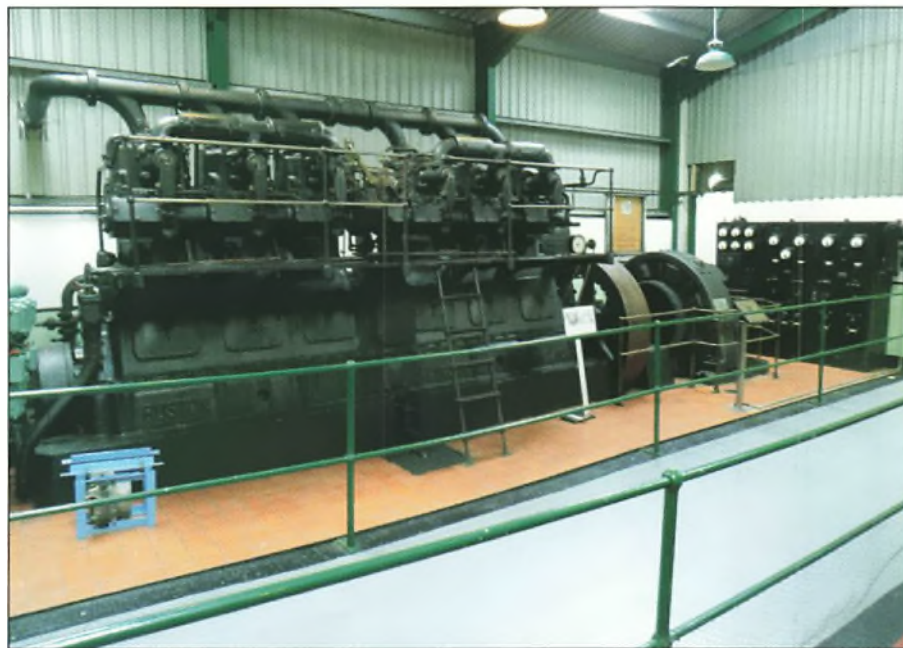
Fig. 1: The six-cylinder Ruston engine and 200kW generator from BBC Moorside Edge Regional Transmitting station.
