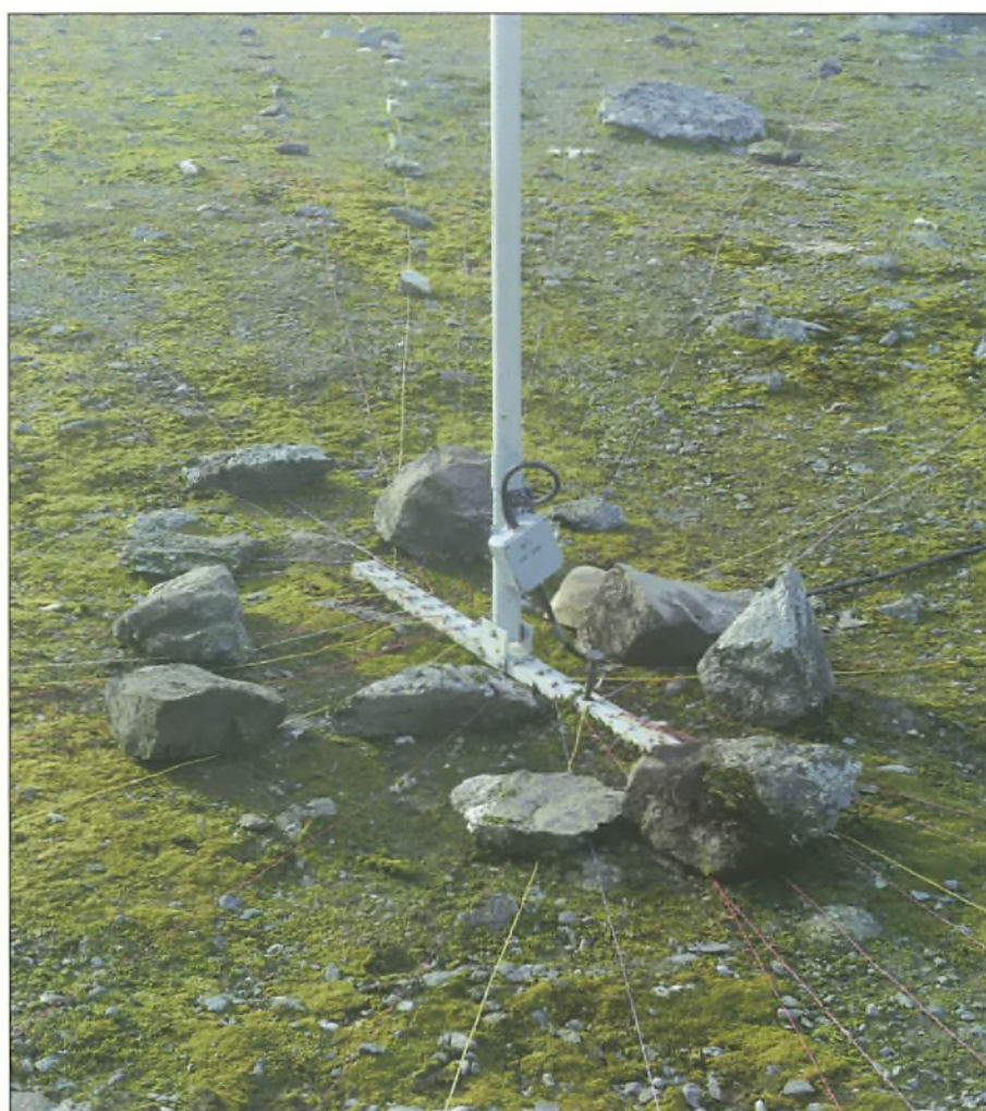
Fig. 2: Base of Battle Creek Special at VP80RK showing radial connections and unun transformer at the antenna feedpoint. (Photo: Ralph KOIR).
