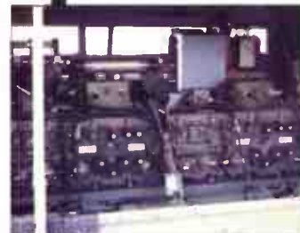
24V C42 radio system in the rear of the FFR Lightweight with the low band Westminster for Ulsternet.
