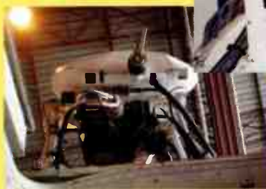
The winch, used by the machine hoist.
