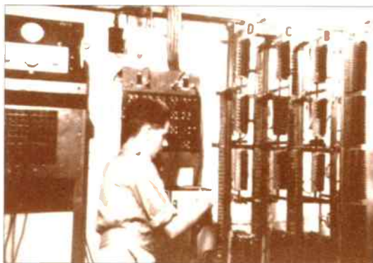
Using a megger to test the high grade lines used to carry the programmes from the studios.
