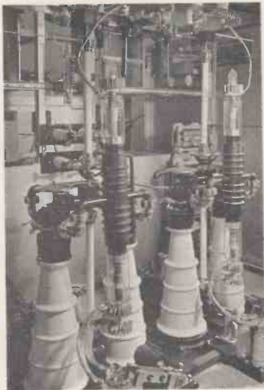
This is the final stage of the modulator unit with mechanical water interlocks which are arranged that the transmitters cannot be switched on until the correct amount of water for valve cooling is flowing.
