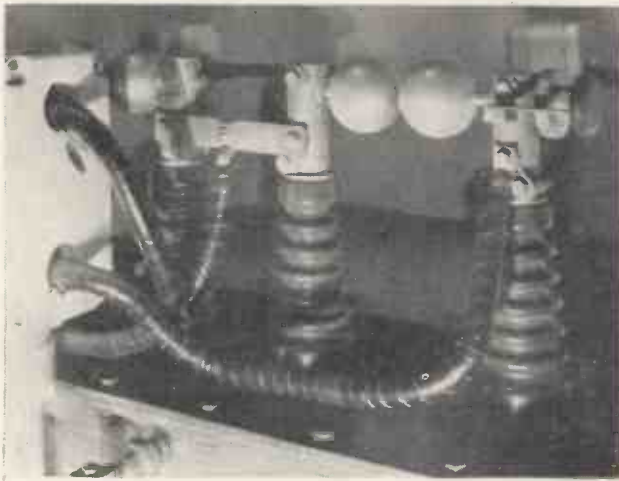
The two balls on a modulation transformer form a safety discharge gap for heavy overloads of current that might otherwise damage valuable equipment.
