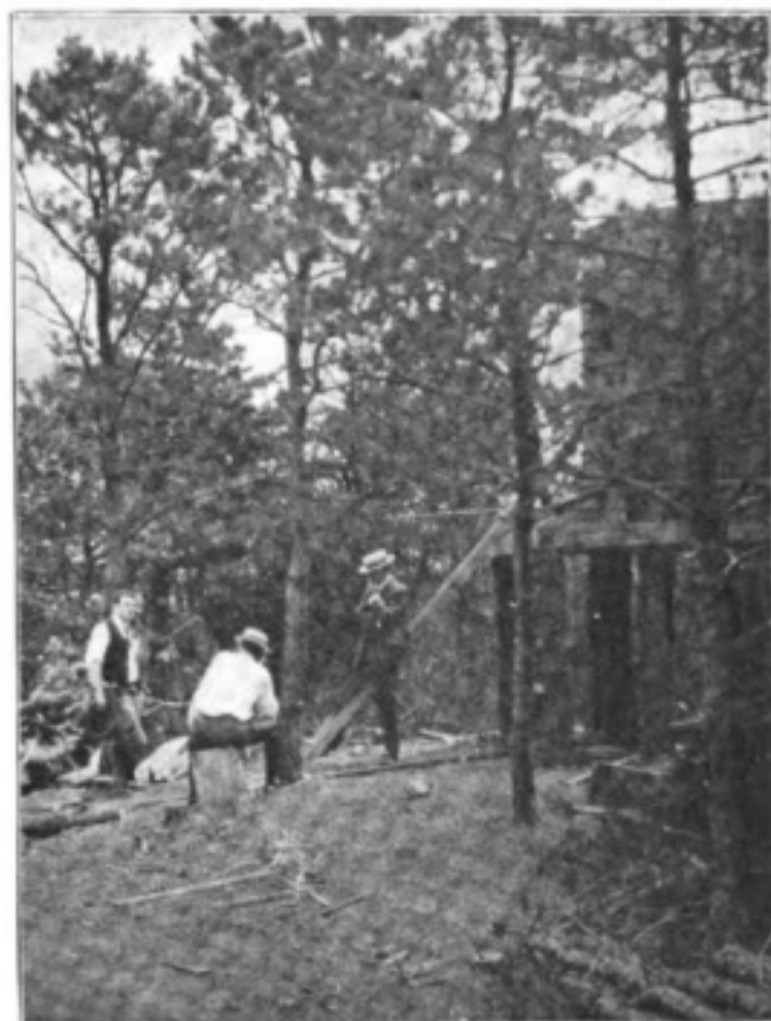
Temporary Water Supply, Chatham Station.
