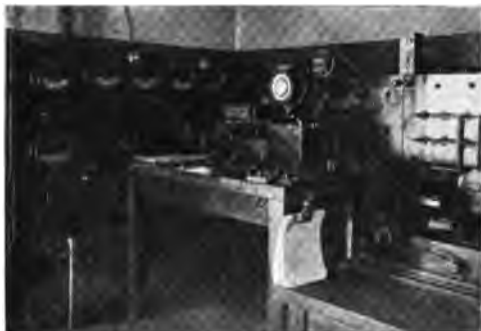
Receiving Instruments and Power Switchboard.
