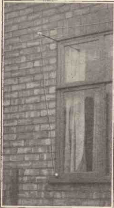
Method of anchoring the lead-in wire in order to prevent swinging, and to remove strain from the terminal of the lead-in insulator.
