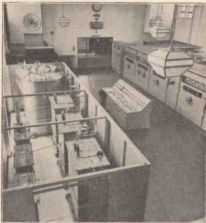
Transmitter Hall as seen from the gallery. The transmitter is on the right and the modulation transformer and plate feed reactors are in the cubicles at the left of the picture.
