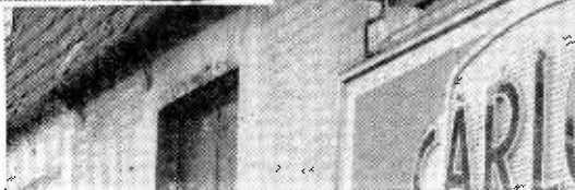
Typical repeater-amplifier mounted on the wall of a radio-and-television dealer's shop in Bedford.
